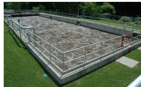
Wastewater Treatment Systems
